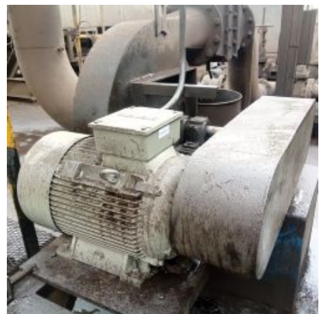
(f) Induced draft fan .
