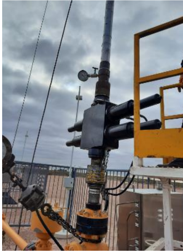
12 Fig.12 BOP (Blow Out Preventer) de Servicios NASER SRL
